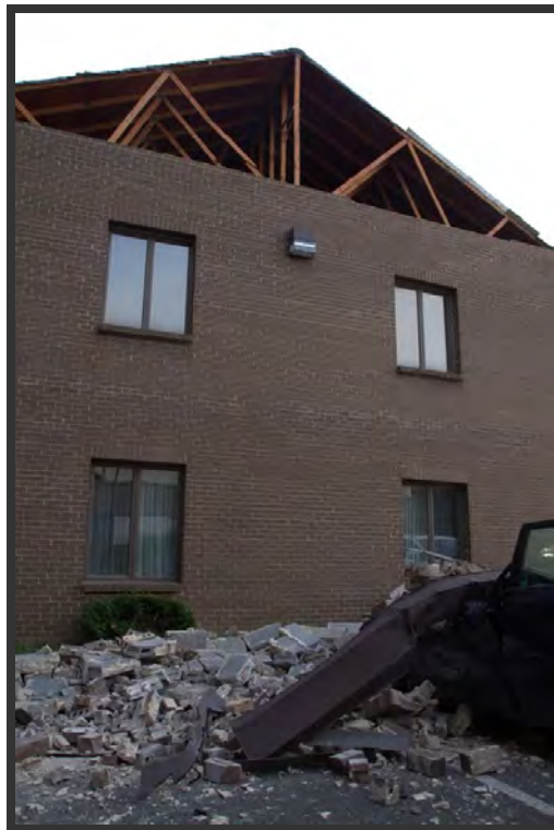
Damage to masonry gable end wall due to moderate ground shaking in a relatively low earthquake hazard region of the U.S. (August 23, 2011 Mineral, VA Earthquake) Source: David Johnston
