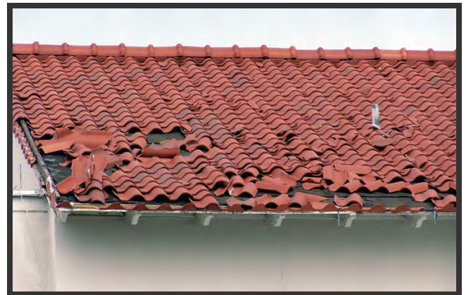
Dislodged roofing tiles due to inadequate anchorage or fastening. Source: FEMA 549
