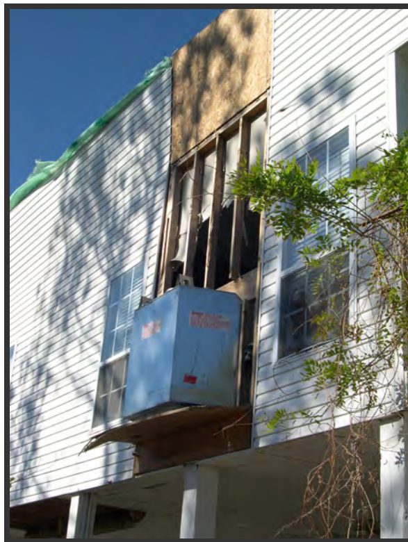
Blown-off light frame chimney (Hurricane Katrina, April 2005)
