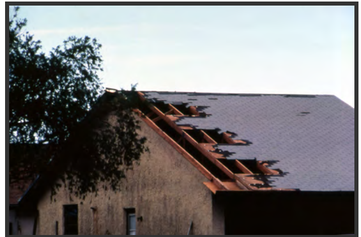
Many homes in Hurricane Andrew experienced low or moderate loss of roof sheathing. Although the rest of the structure may stay intact, the damage from water entry is often extensive. Source: U.S. Department of Housing and Urban Development
