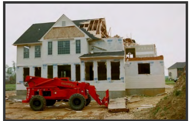
This house probably would have survived a close call from an F-3 tornado had the roof sheathing attachment been enhanced and the uplift load path included additional ties from the wall to the 2 nd floor framing which appears to have been the weak link in this otherwise well-built and code-compliant home. Source: Jay Crandell
