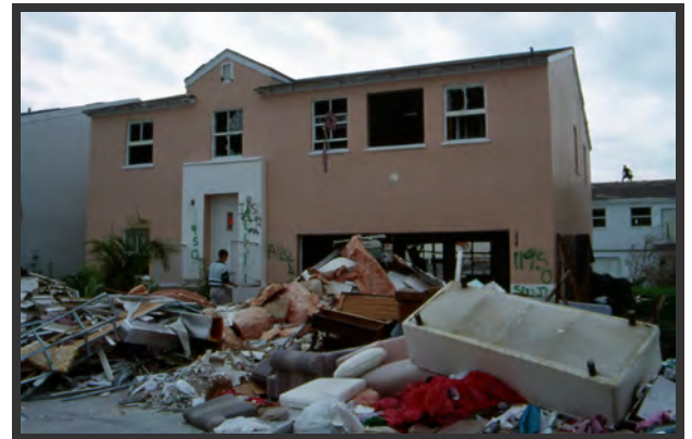
Water soaked contents and destroyed interior of this home were caused in large part by failure of window and door components. Source: U.S. Department of Housing and Urban Development
