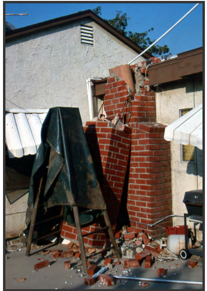
Broken masonry chimney (Northridge Earthquake, 1994)
