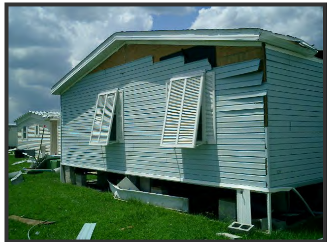
This home suffered loss of siding that could have been avoided with improved siding installation practices. Further, it left the wall open to water damage without the siding or a water-resistant barrier installed underneath.
