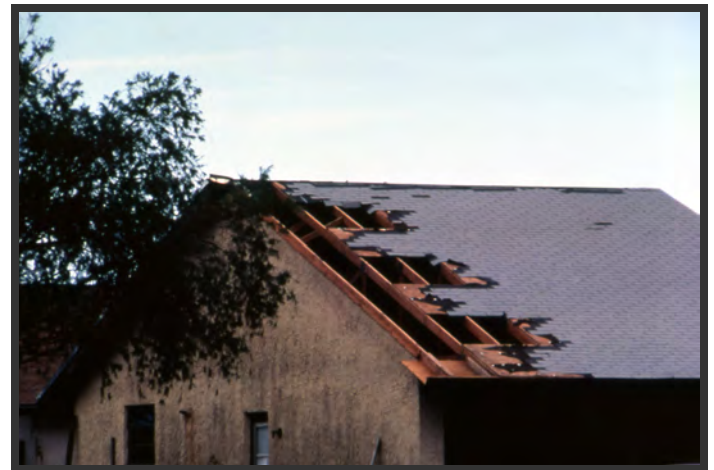
Many homes in Hurricane Andrew experienced loss of gable end overhang framing, often leading to progressive loss of adjacent roof sheathing. Source: U.S. Department of Housing and Urban Development
